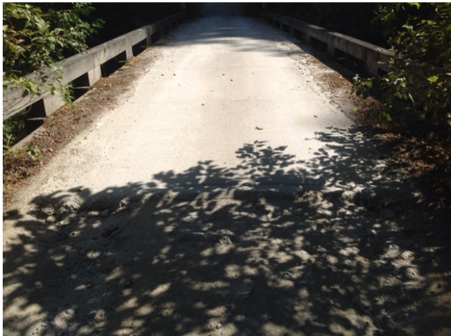
ballast wall damage at road surface
